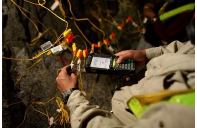
Shotfirer programming the blast. Yellow and red clips indicate the front and rear decks respectively.
